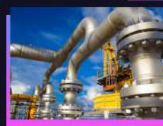
Valves & Valve Automation
